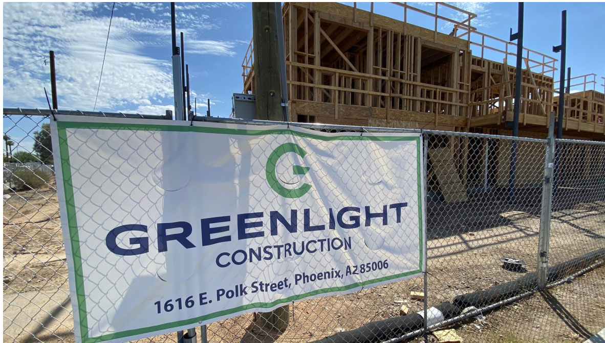
The Streamliner 16th construction site at 16th and Polk streets in Phoenix. Photo: Jeremy Duda/Axios
